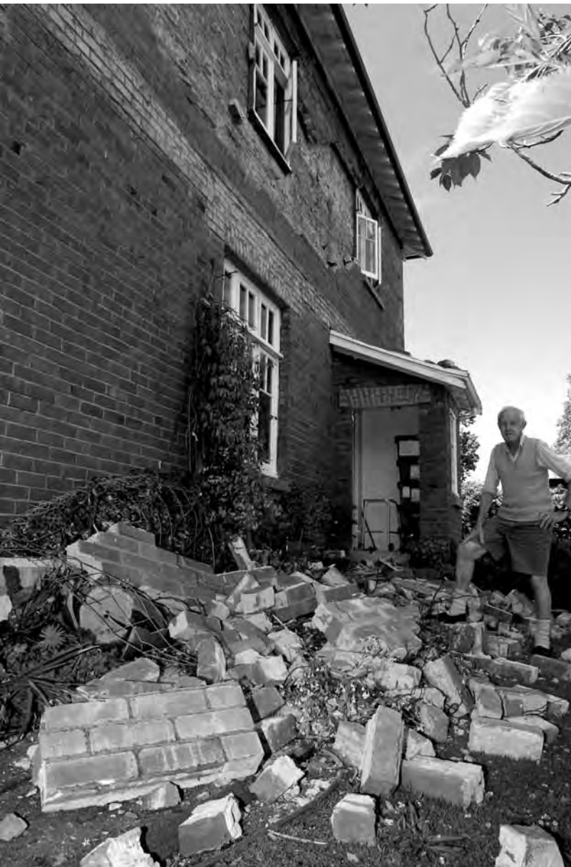
Harold Williams stands among the fallen bricks from the west wall of his house in Gisborne after the magnitude 6.8 earthquake in December 2007. EQC received just over 6,200 claims with costs of around $25 million. Photo courtesy of Gisborne Herald.
